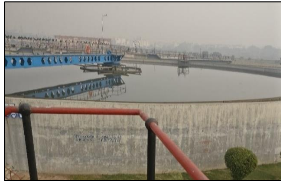
Fig 6: Aeration Tank of Okhla Plant using ASP
