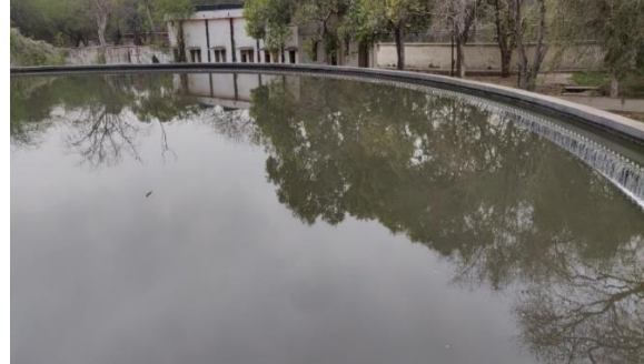
Figure 7: Final Sedimentation Tank
